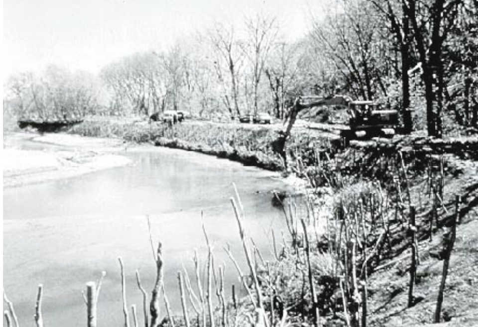
Figure 34. Dormant willow posts, coir geotextile roll, and cedar trees being installed at Court Creek, Illinois, April 1993 (Photo courtesy of Mr. Donald Roseboom, Illinois State Water Survey)
