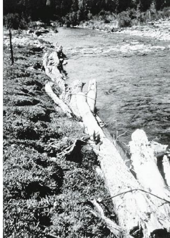
Figure 16. Log revetment, Roaring Fork River, Colorado (Note cable wrapped around logs and buried and secured to dead men in bank)
