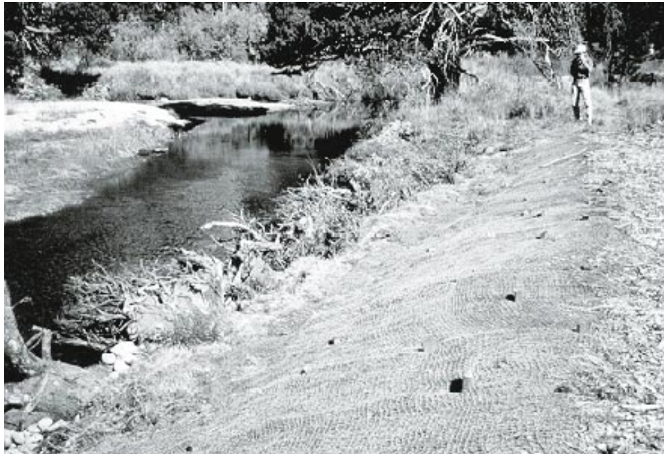
Figure 20. Root wads soon after installation on Upper Truckee River, California, near South Lake Tahoe (Voids within and between root wads are filled with a soil mix and planted with live, vegetative clumps or root pads, such as willow)
