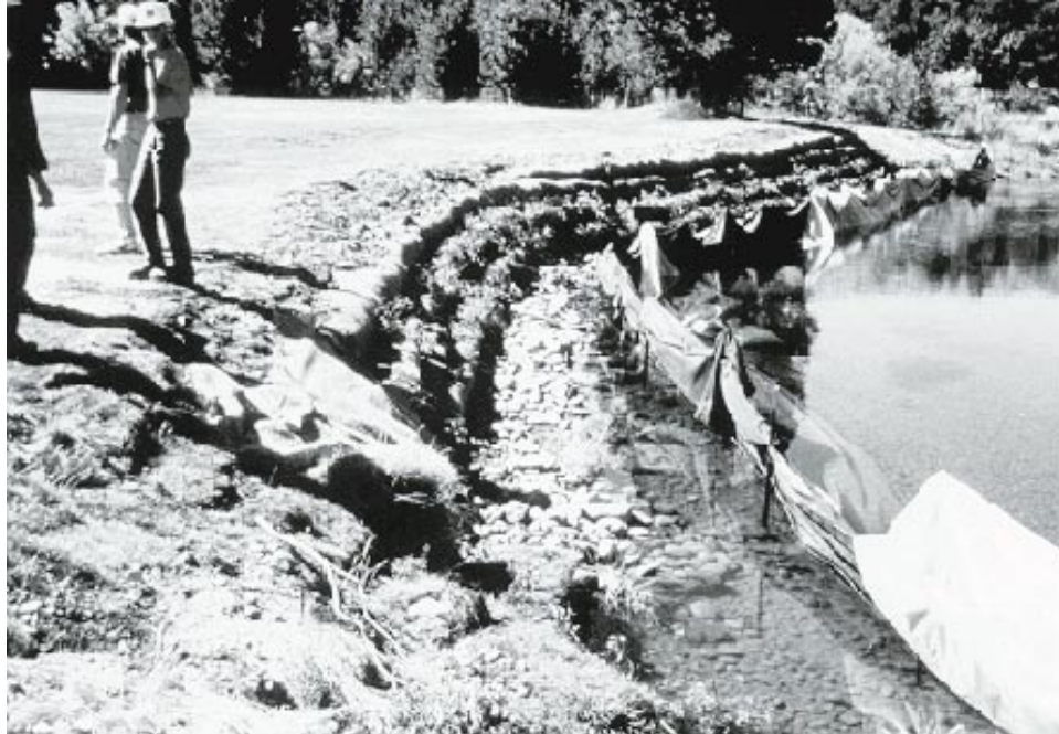
Figure 32. Vegetative geogrid during construction on Upper Truckee River, California, near South Lake Tahoe (Note rock toe that was keyed into channel bed and bank to prevent undercutting. Photo was taken in October 1993)
