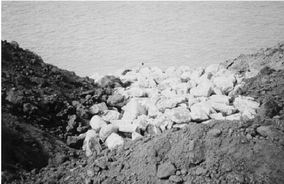
Figure 4. Rock refusal used on an upper Missouri River bioengineering project (Note that it is keyed back into bank to prevent flanking of upper and lower end sections of project)
