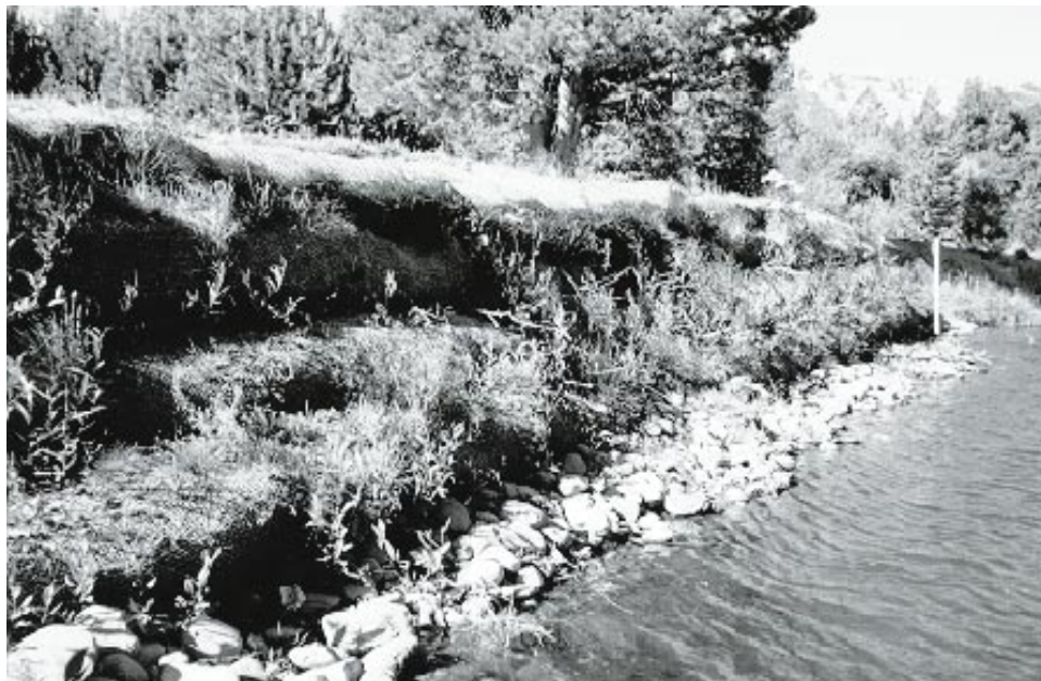
Figure 33. Vegetative geogrid in July 1995, after two growing seasons and an estimated 5-year flood during spring of 1995 (Note that live willow whips that were placed between layers of COIR fabric are sprouting and spreading) (Photo courtesy of Ms. Catherine McDonald, California State Parks)
