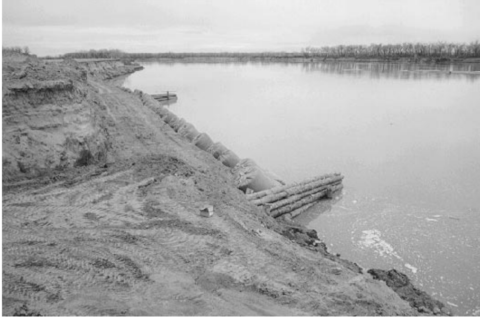
Figure 3. Timber cribs serving as deflection structures on upper Missouri River to direct current away from bank where there are bio-engineering treatments
