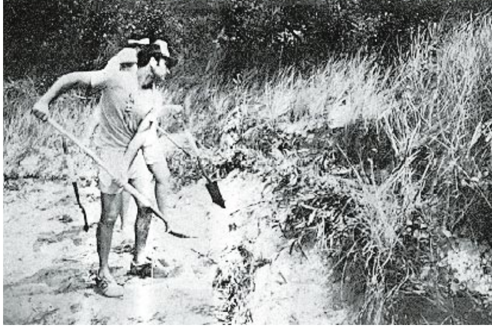
Figure 29. Installed section of brush layering (Note that brush has leaves because of a workshop setting. Normally, brush would be without leaves because of installation during dormant season)
