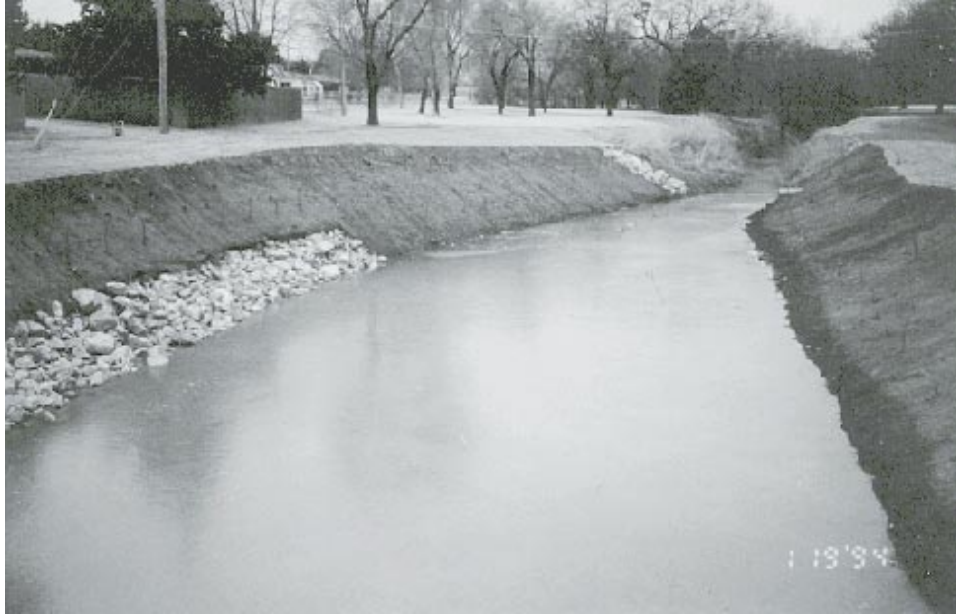
Figure 8. Photo of weighted rock toe revetment extending up the bank (Extends about one-third the distance up the bank. Photo shows stream above low-flow conditions)
